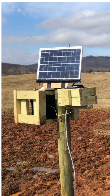
Figure 4: Solar panel and battery at the water troughs
