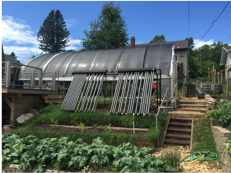
Figure 2: Hoop house with installed solar thermal heat pipe system.
