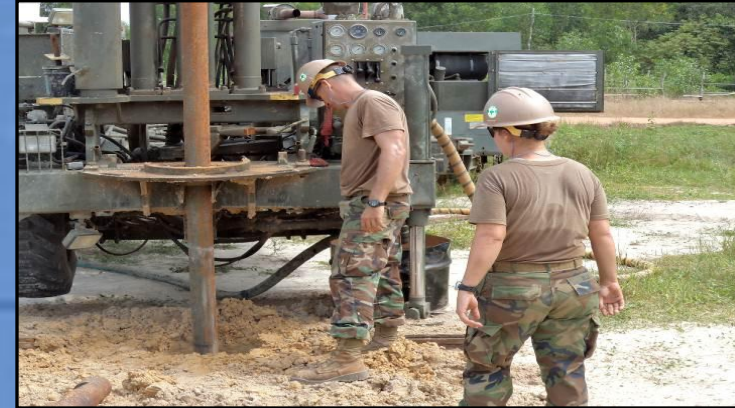
CCAD Cambodia drill pilot hole for surface casing of well at Ream Clinic
