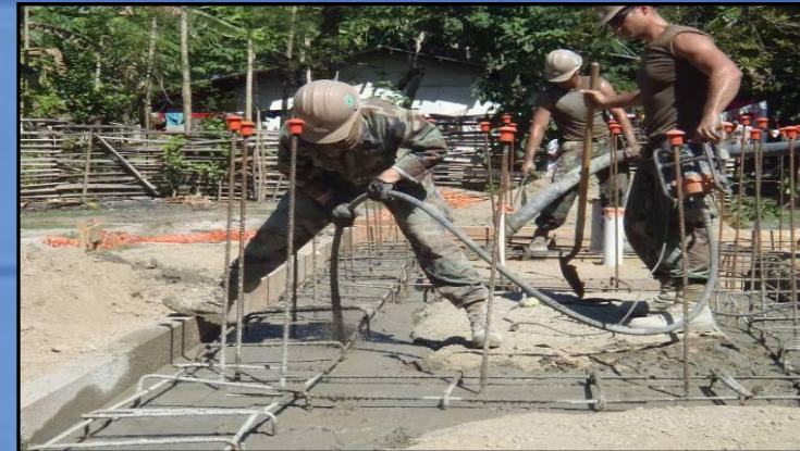
CCAD Timor Leste placing concrete for new schoolhouse construction in Port Hera
