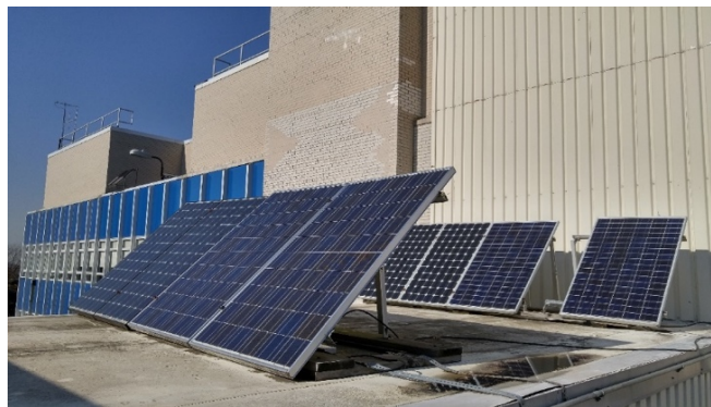
Figure 1 Picture of installed solar modules on the roof of the Technology Building at QCC
