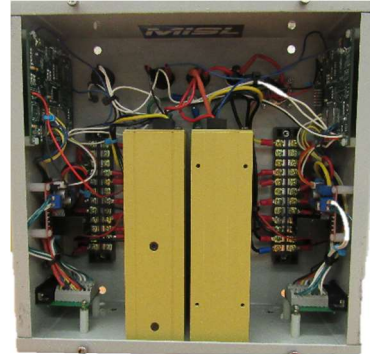
Figure 3. STRATA 1 Control and Monitoring Unit.
