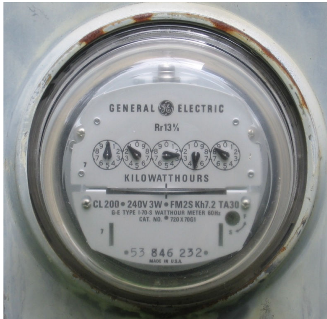
Figure 2. GE CL200 Watt-Hour Meter
