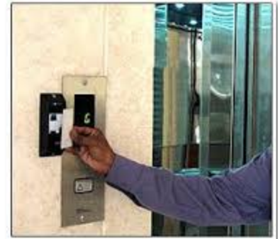
electronic access controls
