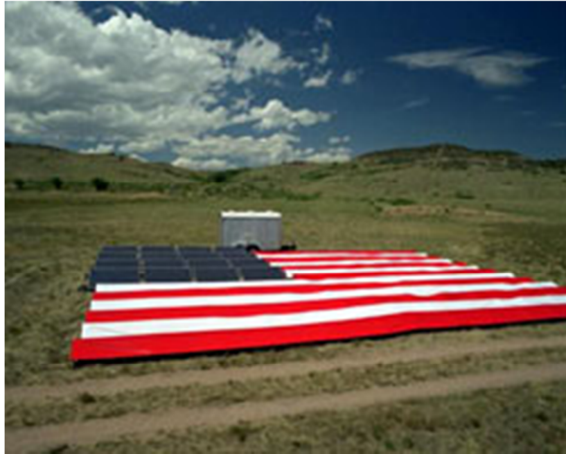
Figure 2: NREL Solar Independence Photovoltaic System. Storage trailer in background with photovoltaic panel array in upper left of flag demonstration 6 .
