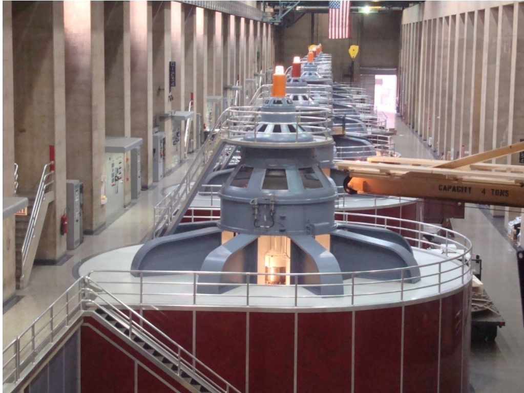
Inside the belly of The Hoover Dam power generator housing.
