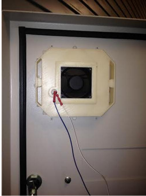
Figure 3. Cooling fan addition
