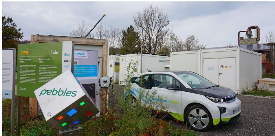
Figure 11. Lithium-ion battery units and community electric vehicles are managed as part of the PEBBLES peer-to-peer energy trading system in Wildpoldsried, Germany
