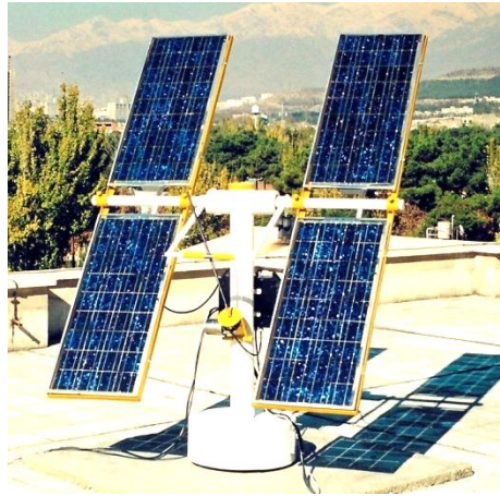
Fig.8 Two-axis photovoltaic tracker implemented by solar project team [2]
