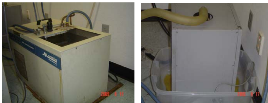
Fig. 6: Left - Water cooler, and Right - Rotary Pump
