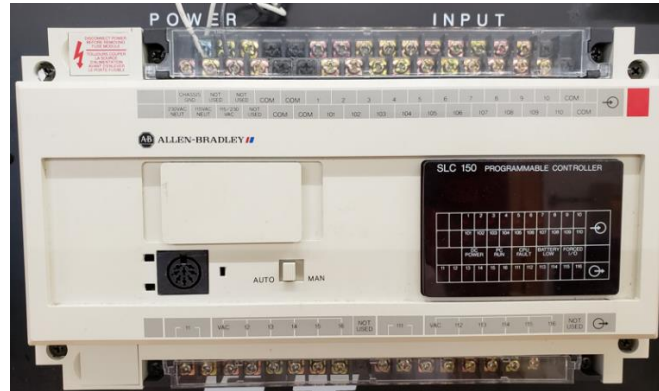
Figure 2. Allen-Bradley SLC 150 PLC
