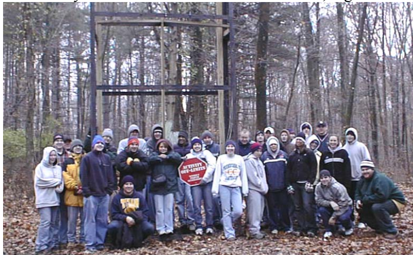
Figure 1. MAE and HSS students gather in front of the wall skeleton after spending the day tearing down the old wall.
