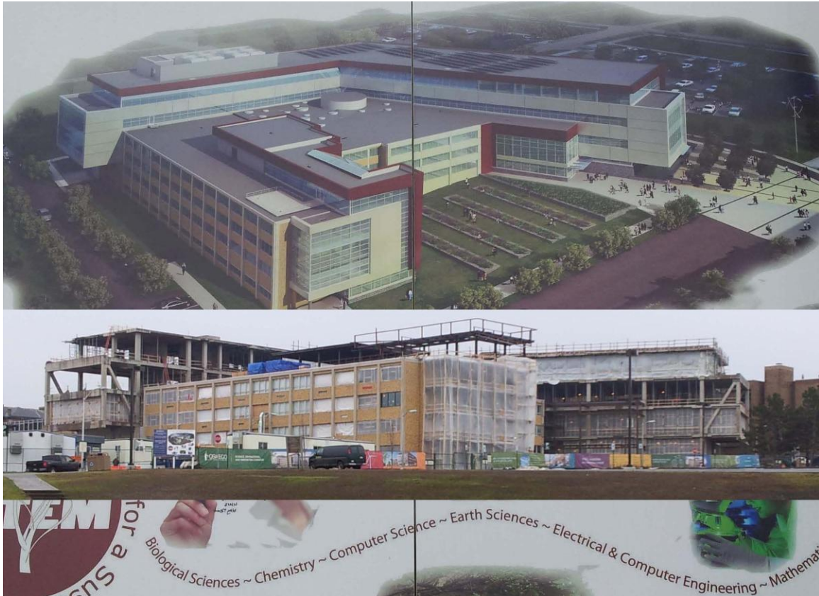
Fig. 1 The Science and Engineering Complex : current construction status and planned final appearance.
