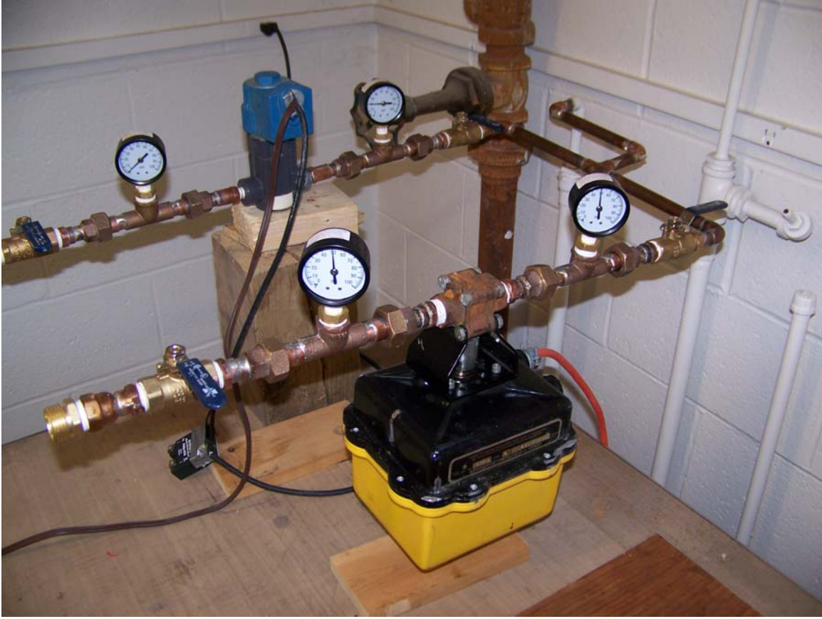
Figure 1. Flow Control Valves
