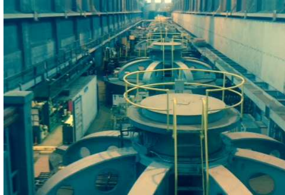
Figure 3. Hyrdo Turbines at Ohio Falls Generating Station.
