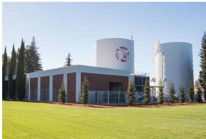
Figure 3: Thermal Energy Storage Tank at the CSU Chico Central Utility Plant
