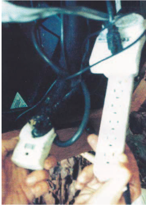
Figure 4. Two power strips – The left one is completely burned; the right one is not changed.
