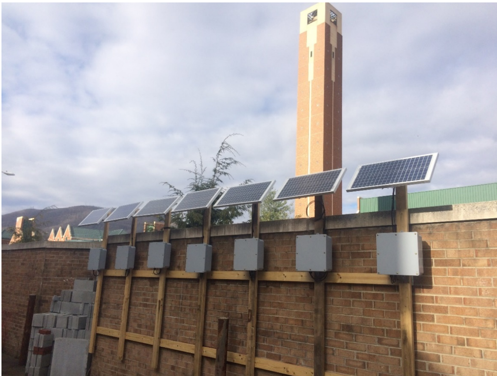
Street Lamps deployed for testing
