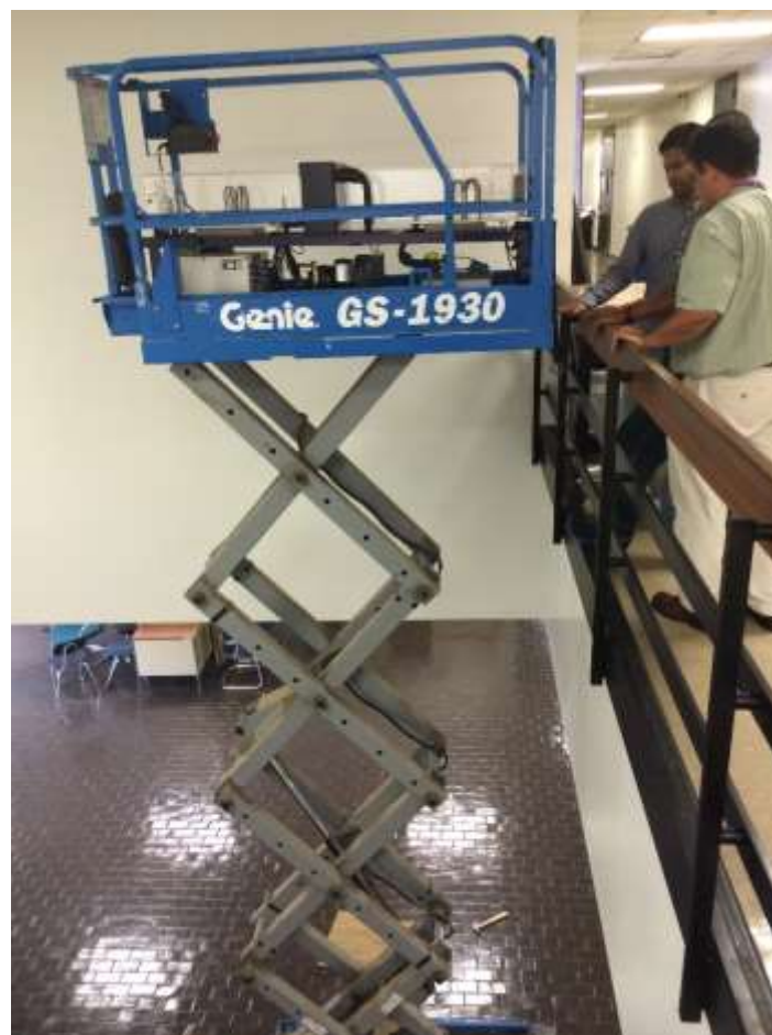
Figure 2. Lab Establishment Challenges: Moving the Air Conditioning Unit to the Second Floor without Tilting
