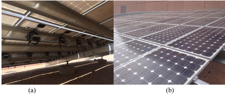
Fig.1: The Cyber physical (CPS) system allowing transmission of analytics and enabling the control of the system from remote sites. The figure shows (a) Solar array research facility with SMDs attached on each panel. (b) The SenSIP solar array facility. The educational value of this CPS facility is that students can learn about sensors and sensor fusion, the use of machine learning to optimize solar energy production.
