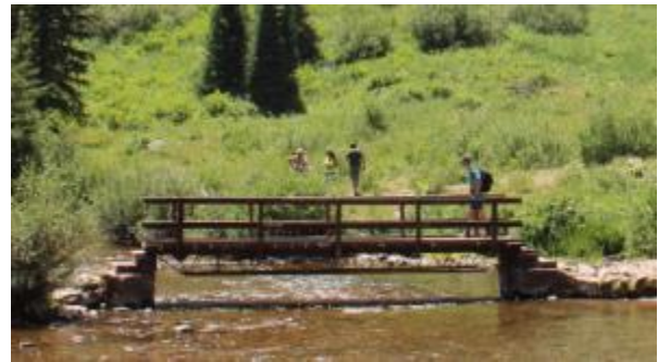
Figure 5. Open web steel joist bridge type located at Maroon Bells. Note the cord and web members beneath the bridge
