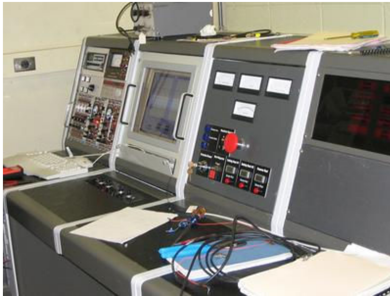
Figure 1 The Texas A&M AGN 201 Reactor Control Console
