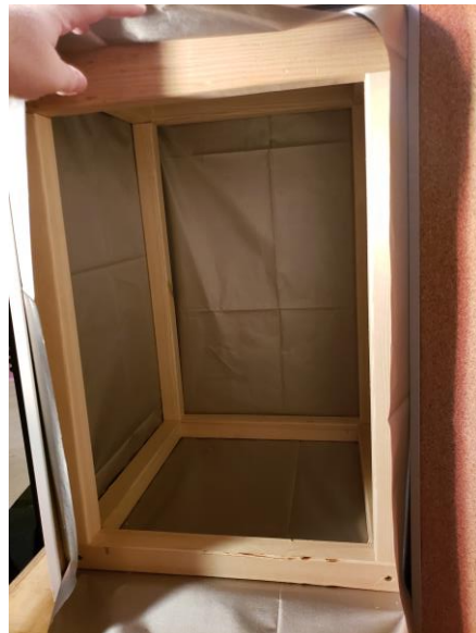
Figure 5: Supports Installed in the Cabinet
