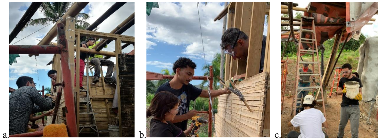
Figure 3. Bamboo Experience. (a).Working on an outdoor bathroom. (b) Building a lath wall using bamboo “esterilla”. (c) Bringing a bucket filled with cement to fill holes in bamboo poles near joints.
