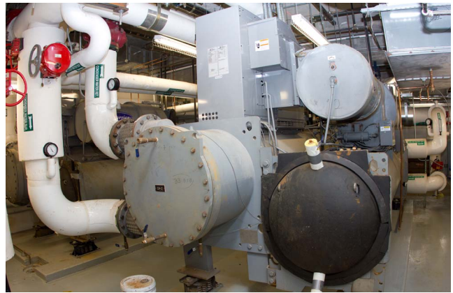
Fig. 3. Centrifugal Chiller. Students visit the chiller mechanical room during building tours.
