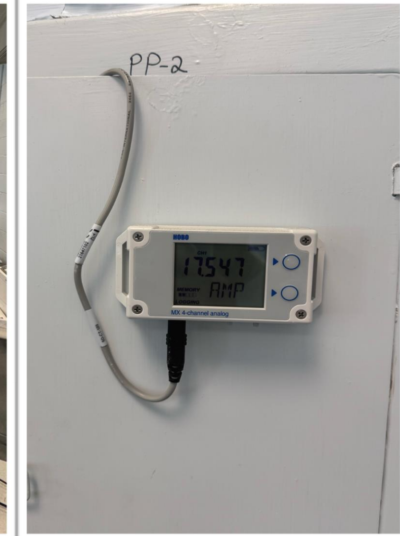
Figure 3: Hobo Data Logger
