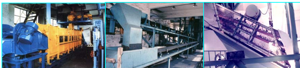
FIG 6 Pilot systems of fluidization dry coal separation and sieving
