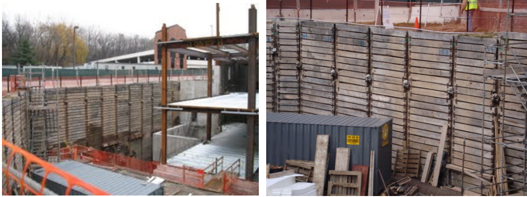
Figure 24. Soldier piles and lagging with soil anchors and some waler blocks (Photos used by permission)
