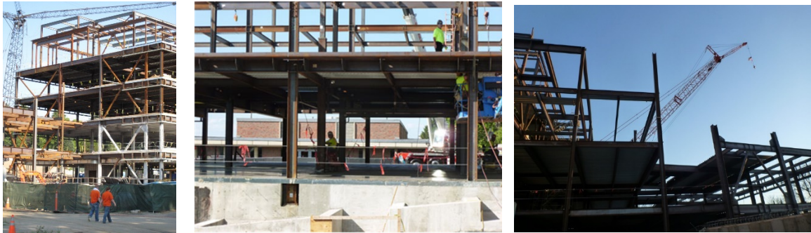
Figure 3. Ideal stage of construction for steel design course (Photos used by permission)
