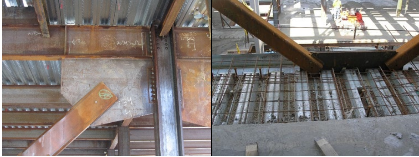
Figure 5) Braces and their connections (Photos used by permission)
