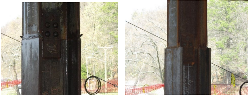
Figure 6. Column splices: similar members (left) dissimilar members (right) (Photos used by permission)
