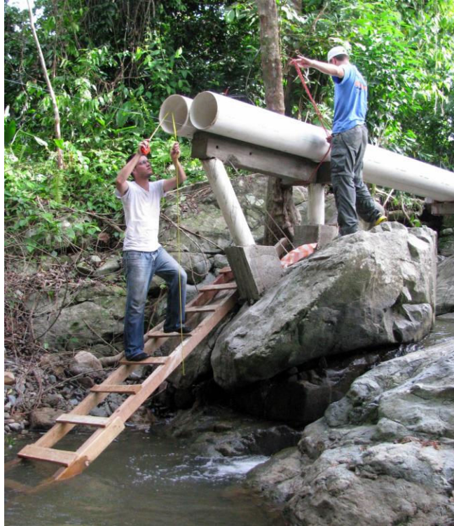
Figure 3: The construction of the piping system to deliver water to the generator.
