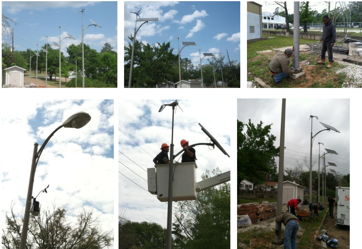
Figure 4. Solar Photovoltaic Lab and project environment
