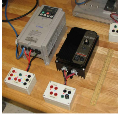
Figure 5. Connection boxes for drives.
