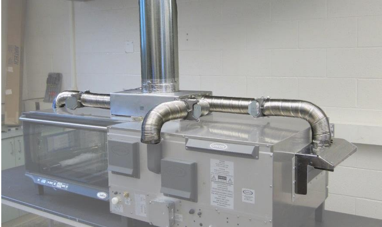
Figure 9. Ventilation system designed for POS capture at each end of the ovens and exhaust vents
