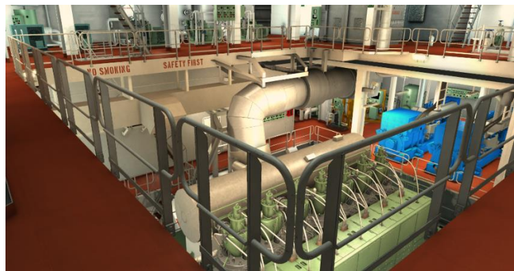
Fig. 5. TAMUG MARE VR machinery space.
