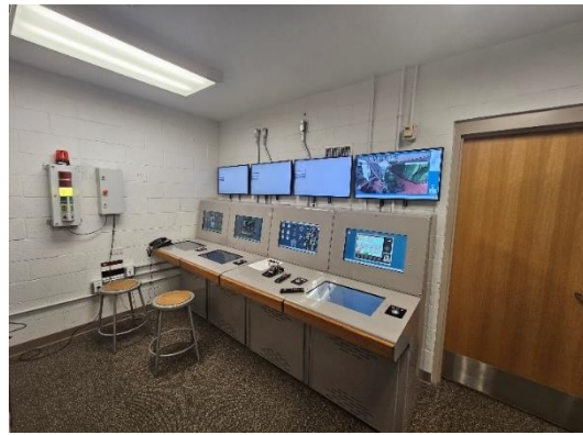
Fig. 4. ERS 2 FMS engine control room.
