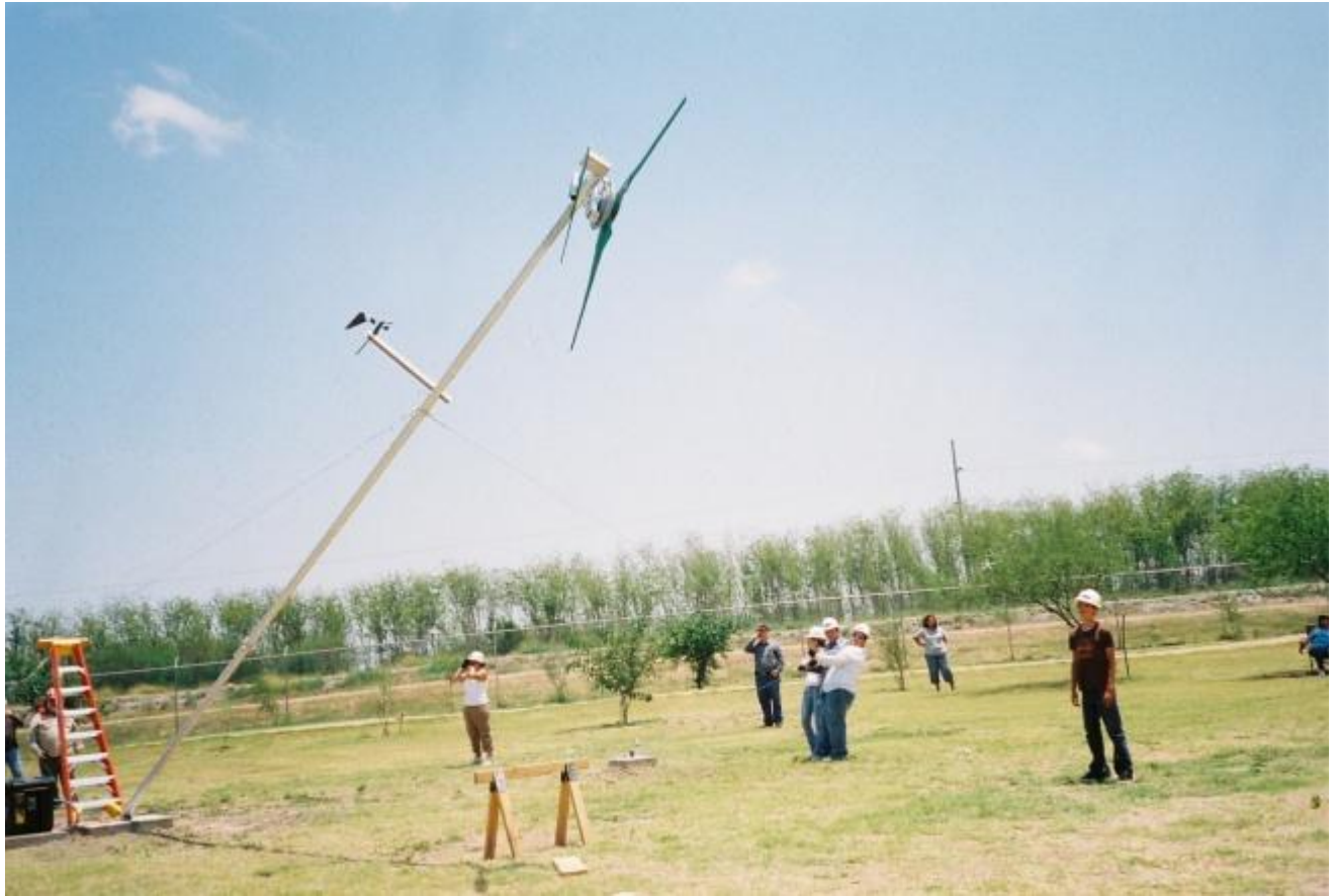
High School Students Erecting Their Wind Turbine, Complete with Data Acquisition System
