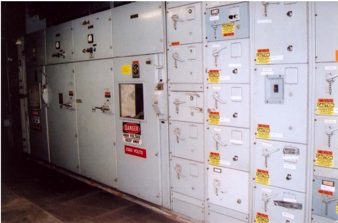
Figure 4: A sampling of the more than 300 electrical closets at a very large food warehouse in New Jersey.
