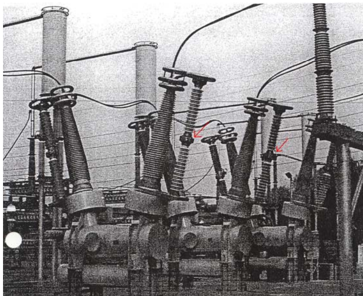
Figure 1: 3-phase circuit breaker, 250,000 Volts. Note – Capacitor that caused accident labeled with arrow.
