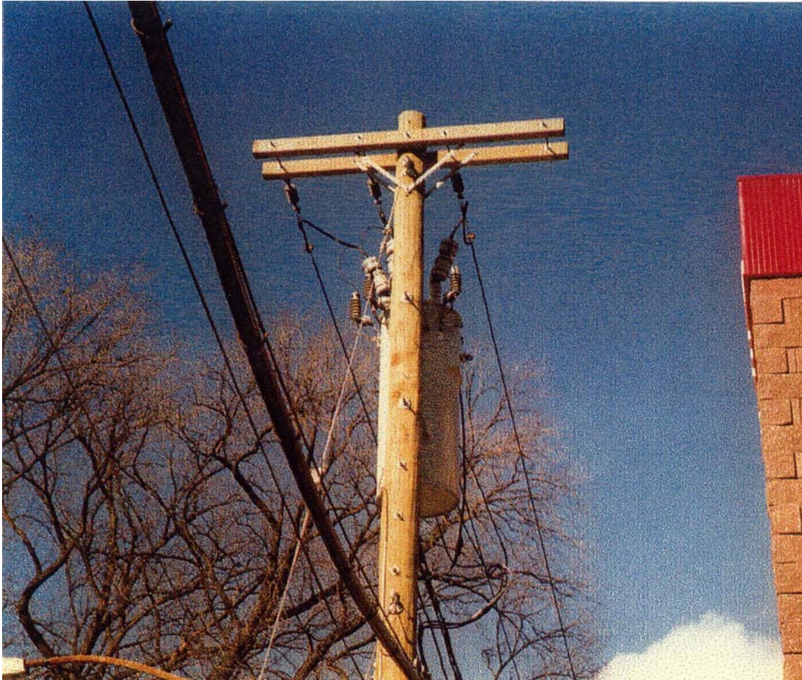
Figure 2: Telephone pole with 3-phase 13,000 Volt power cable near building (right) where accident occurred.
