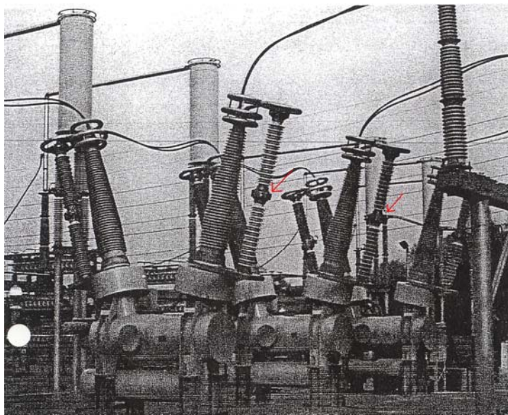
Figure 1: 3-phase circuit breaker, 250,000 Volts. Note – Capacitor that caused accident labeled with arrow.
