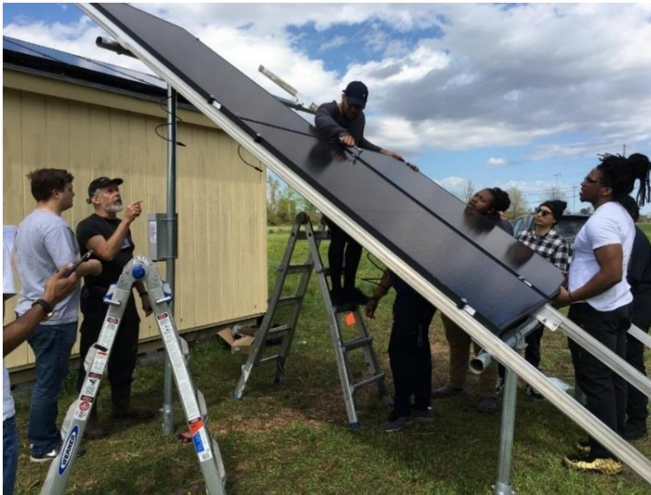
Photo 2. Students installing a 1300W ground mount photovoltaic (PV) system at the renewable energy demonstration and training site
