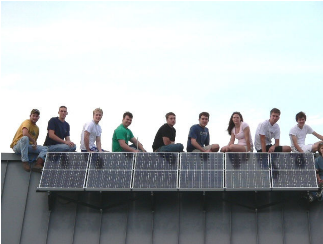
Figure 1. Students pose for a picture after installing six BP7185 185W (peak) PV modules and a powder-coated steel mounting structure on the Museum’s standing-seam roof.
