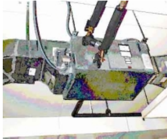
Figure 6. Fresh air intake coil assembly suspended from ceiling – coil inlet and outlet piping along with the condensate drain is shown.
