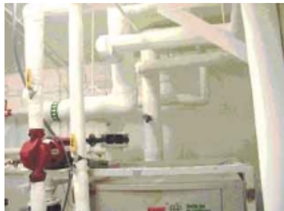
Figure 5. Insulated piping installed by inmate labor at Northwest Tennessee Correctional Facility.
