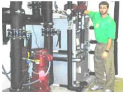
Figure 4. Student beside two geothermal water source heat pumps in Guild 5.
