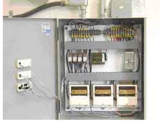
Figure 9. View inside of control panel after installation in prison facility.
