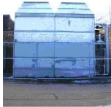
Figure 2. Cooling towers used in the existing central loop system.
