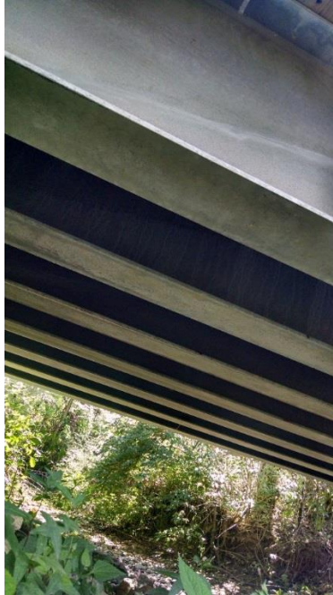
Figure 3 I-beam Bed of the Truss Bridge as Viewed from the Bottom of the Bridge
