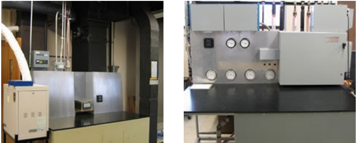
Figure 1. Direct access to HVAC equipment provides little insight to equipment performance.
