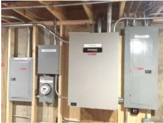
Figure-1 Electrical Control Room
