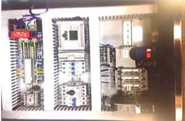
Figure 3 Completed Control Box
