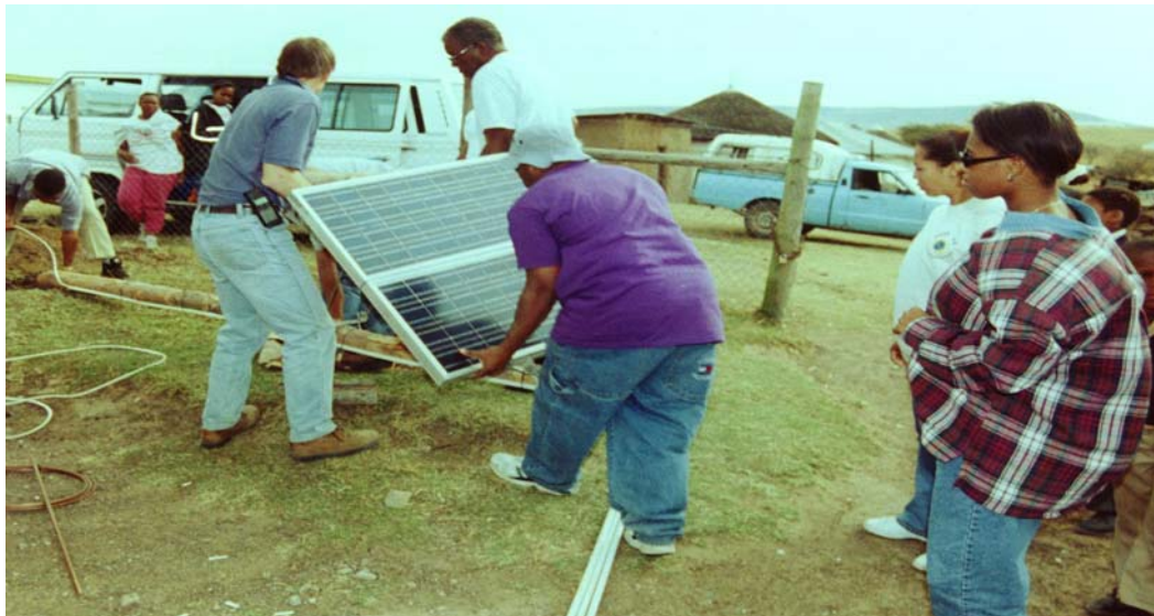
Figure 8: REEP Students and Staff installing the 100-Watt Solar Electric System in South Africa
