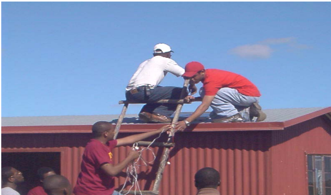
Figure 13: Installing Solar Electric System on the Roof of a Pre-School in South Africa
