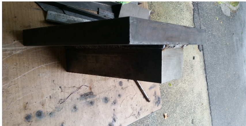
Figure B2 – Shown is the attachment via arc welding of the base block and clamping plate
