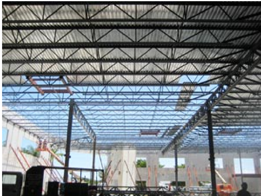
Figure 3 – Typical Open-Web Steel Joist Used in a Roof System (Courtesy: Steel Joist Institute http://steeljoist.org )
