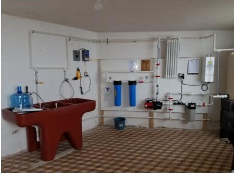
Fig. 2. Water purification system in Guatemala.
