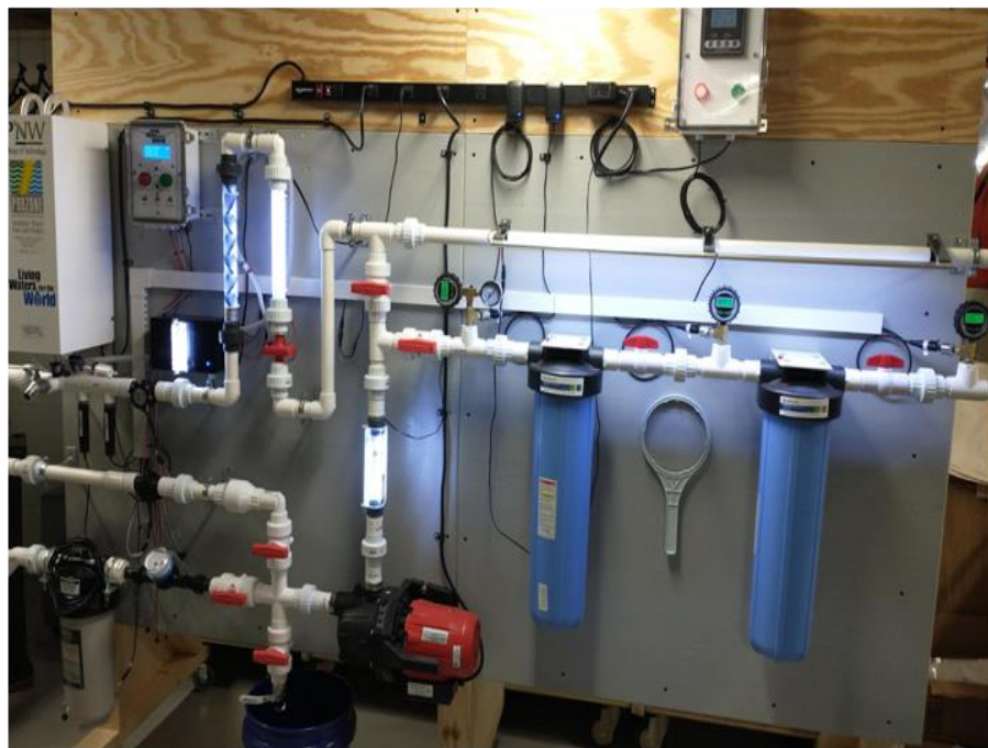
Fig. 3. Water purification test model in CID building at PNW.
