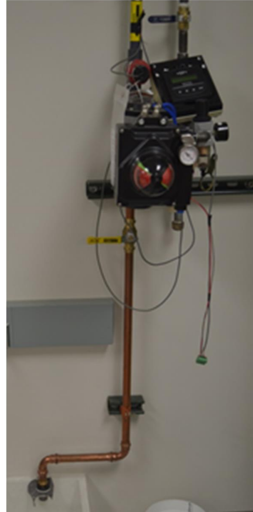
Fig. 6. Abandoned flow control valve.
